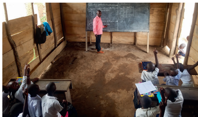
There wasn't enough wood to finish one of the walls in the new school. When it rains, it gets wet in the classroom.
